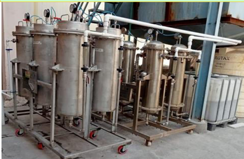
75-100 KLD Industrial plant BARC demonstration facility at JSC (>10,00,000 L) RajKaj Ref No.: 12131006
