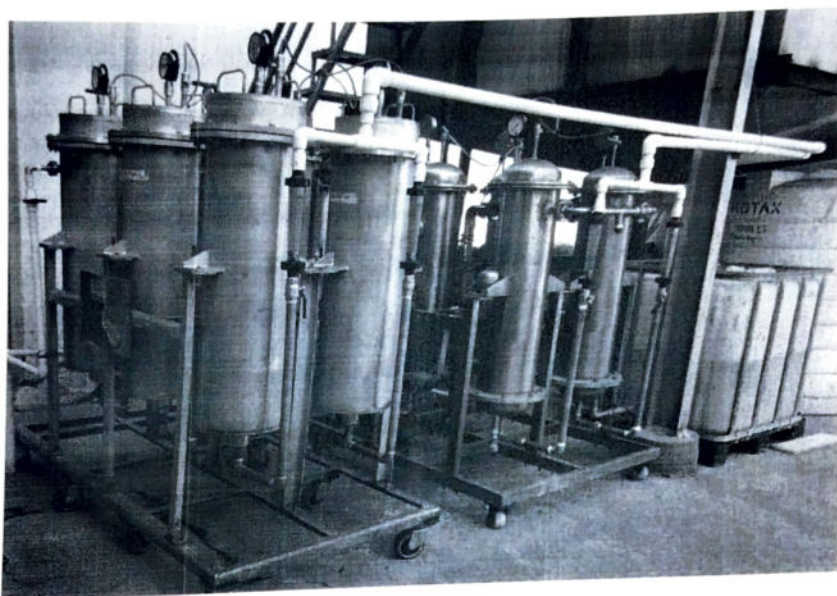
75 KLD RAD-TED plant
